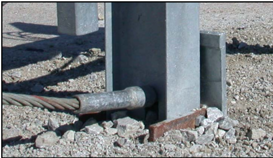
Figure 18. Cable Anchor Assembly at Post #1 for BEAT-BP
